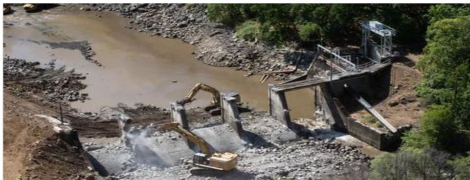
Down comes Copco No. 2. Destruction of Hydroelectric Facility on the Klamath River is underway.
