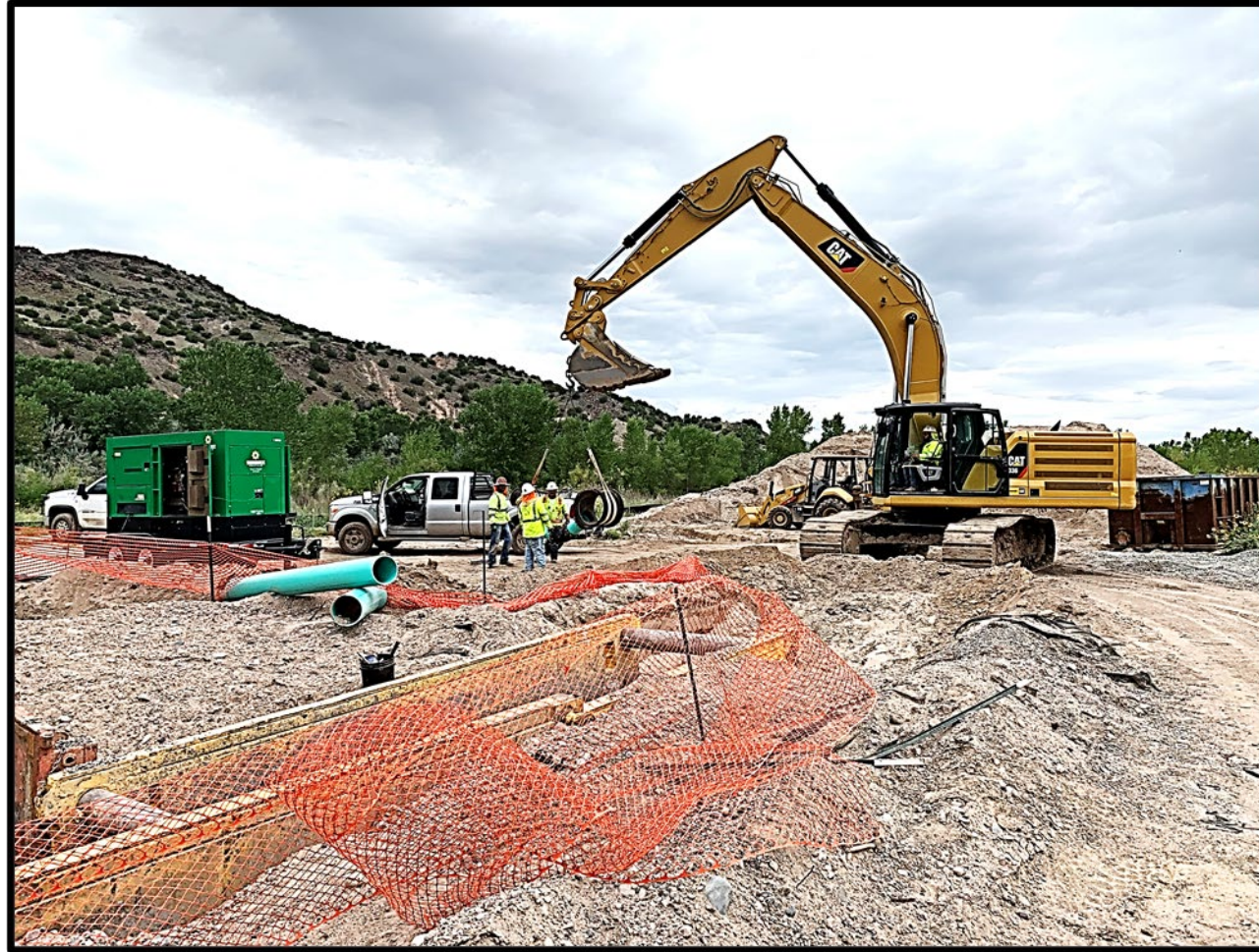
Photo: Reclamation-funded construction underway on the Pojoaque Basin Regional Water System (New Mexico), September 2021.
