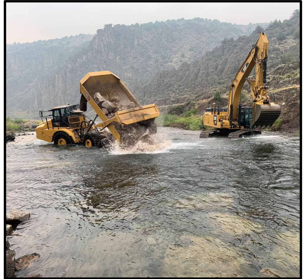
Photo: Reclamation constructing a new riffle in the Teton River downstream of remnants of Linderman Dam (Idaho) to improve habitat, resolve a public safety issue and provide reliable irrigation, October 2021.
