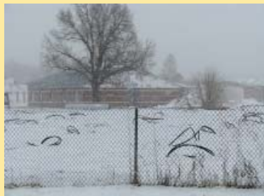
Tubes linking the ground source heat pump wells next to the new Pine Ridge School dormitory in South Dakota emerge through a spring 2009 snow.
