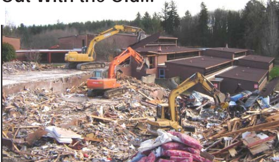
The dormitory cottages at Chemawa Indian School in Oregon are demolished in January. A new 86,400 square foot dorm, which includes a commons area (right), now houses 400 students. The OFMC Project Manager is Phil Asmus.
