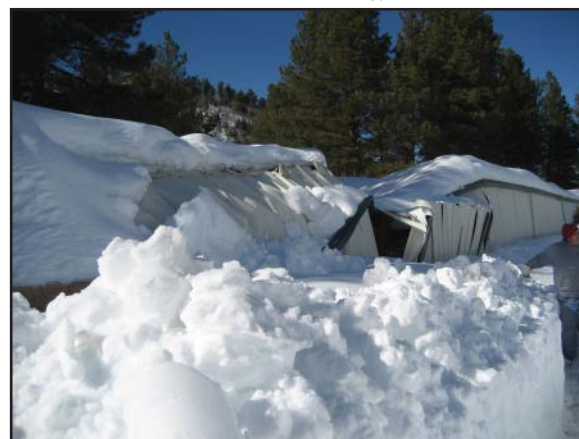
This building at the McNary location of the Fort Apache Agency in Arizona collapsed in January.
