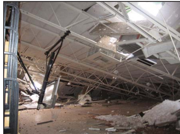
The gym roof collapsed in January at Shonto Preparatory School in Arizona. The gym was built in 1966.
