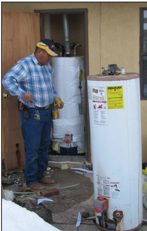
Michael Smith installs a new water heater at his Mescalero home in February.
