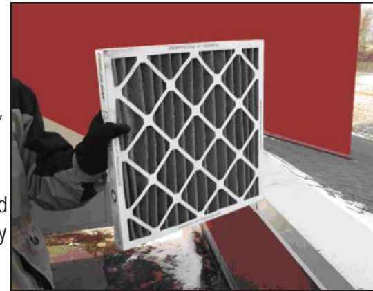
Dirty air filter at Nay Ah Shing.
