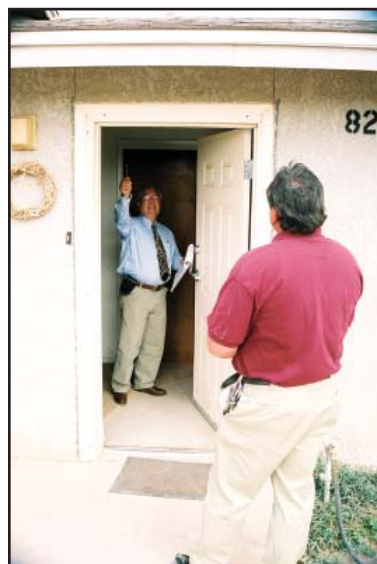
Employee housing assessment inspector Michael Morrison examines a door frame of a home at Tohono O'odham High School in Arizona while Papago Agency Quarters Manager Lee Ivey looks on.
