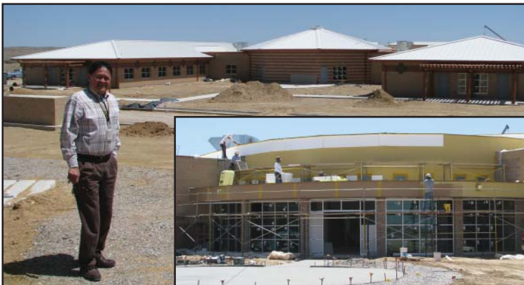
Pueblo Pintado Community School Principal Notah Benally visits the school's new dormitory, while workers prepare the school gymnasium entrance (inset).
