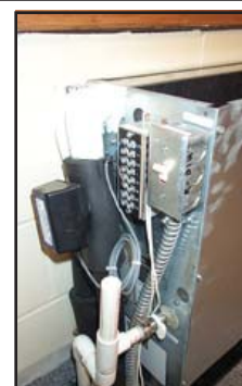
The closed loop system (top) at Circle of Nations sends a water/glycol mixture through polyethylene piping (now covered over). The earth-warmed/cooled mixture is circulated by pumps (middle) to a classroom heat pump (below) where it assists in heating or cooling.
