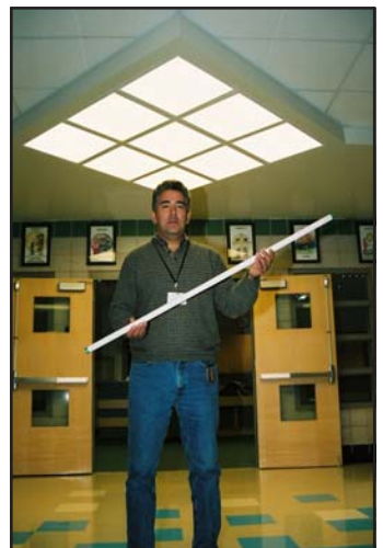
Dan Anderson, Fond du Lac's facility manager, ensures that energy efficient fluorescent bulbs are used.
