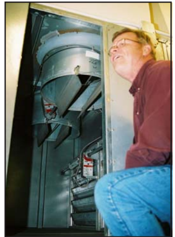
Lafontaine inspects vents for proper response to his electronic settings.
