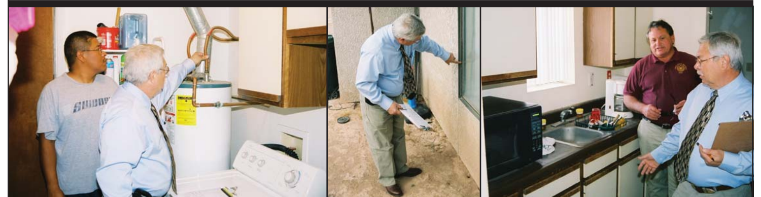
Morrison and Antone check the home's water heater and utility room hook ups (left). Windows have been damaged (center) due to multiple break-ins by illegal aliens seeking food and water while traveling through the desert near the Tohono O'odham High School employee housing neighborhood. Morrison and Ivey discuss the condition of a kitchen (right).
