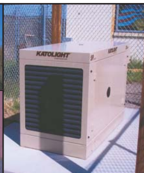
Through Pub. L. 93-638, the BIA funded a propane-fueled, back-up generator (above), rated at 25 KW.
