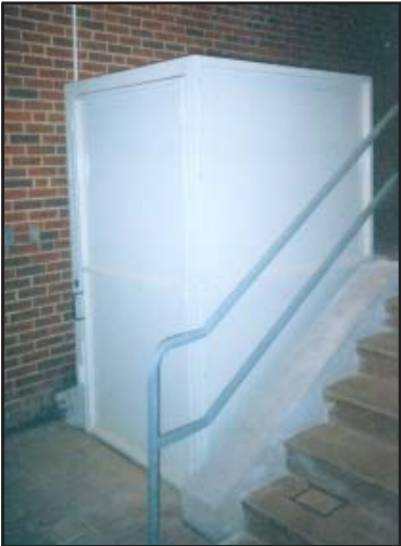
New elevator lift at Eagle Butte.
