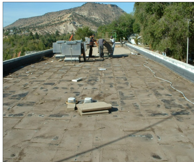
A roof is being repaired at the Warm Springs Detention Center, OR.
