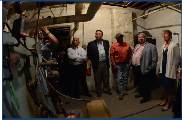
Secretary Jewell is shown an outdated and often broken boiler located in a converted coal chute at Crystal Boarding School in New Mexico. The room is cloaked in asbestos and this makes repairs to the boiler extremely difficult.
