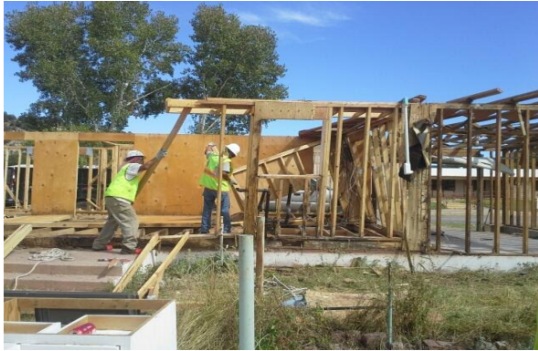
John F. Kennedy Day School Quarters Under Construction In Cedar Creek, AZ
