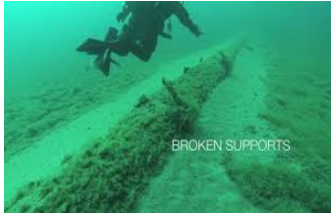
View of Line 5 pipeline in Straits of Mackinac
