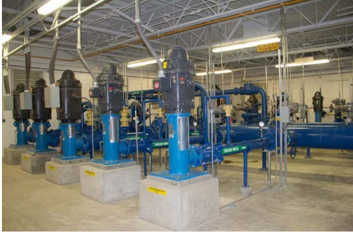
Fort Peck Water System, Fort Peck Montana
