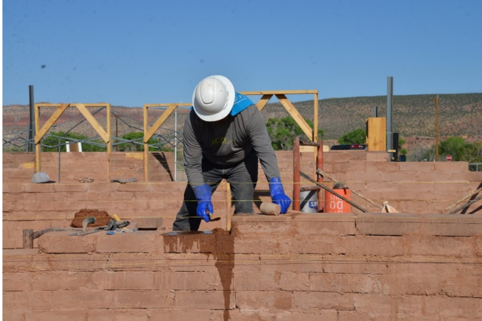
High Performance Adobe crew member laying blocks for the first demonstration home at Pueblo Place, Jemez Pueblo.
