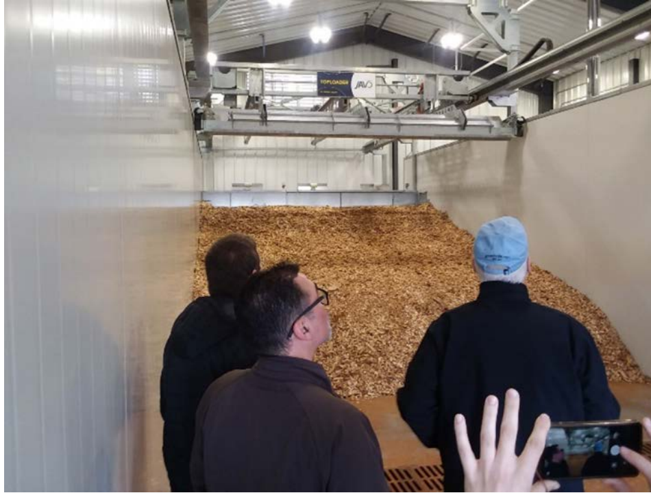
Wood chip storage for the Fond du Lac woody biomass district heating facility, commissioned in April 2018.
